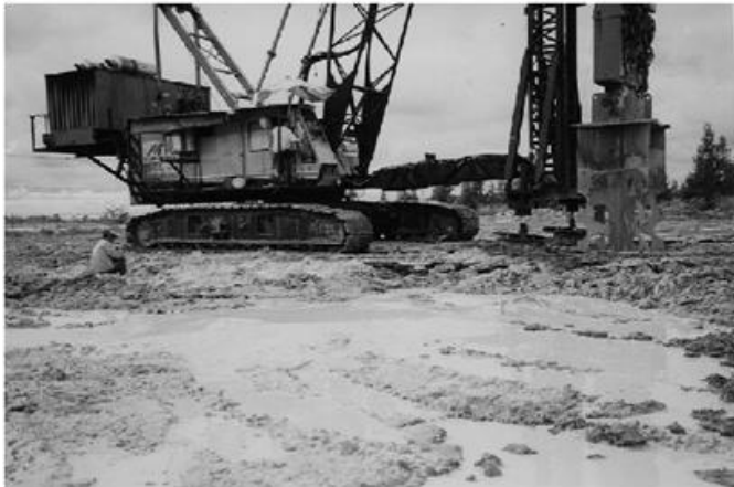
Figure 4.13 Liquefaction of water-saturated sand during the initial phase of compaction. Note that the groundwater level is 4.5 m below the ground surface.
